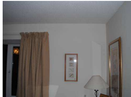
Cold air movement behind walls
