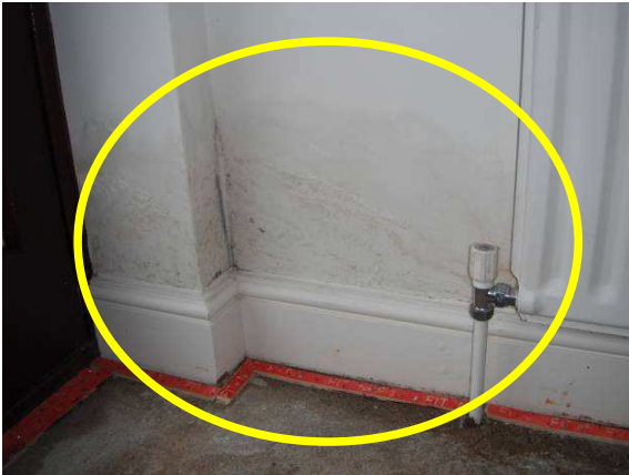
Fig.1 Water Damage at Base of Wall in Hall
