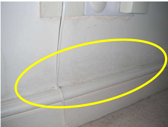
Fig.3 Water Damage at Base of Wall in Hall
