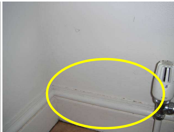
Fig.4 Water Damage at Base of Wall in Dining Room
