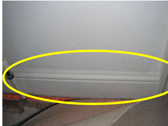
Fig.2 Water Damage at Base of Wall in Hall
