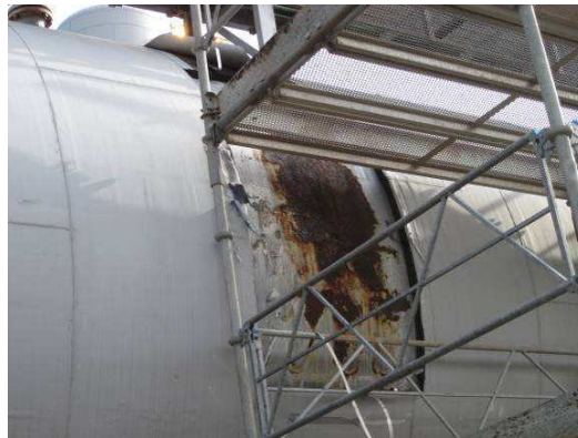
Fig.2 Digital Image Showing Section of Removed Insulation with Clear Corrosion Having Commenced
